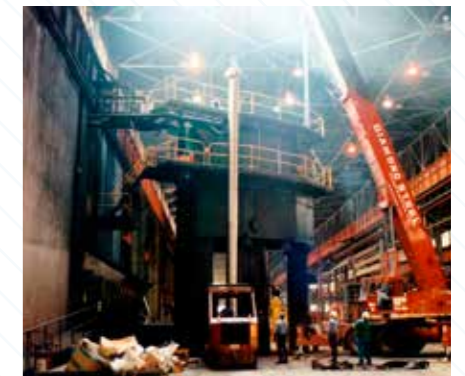
The world's largest bolt-style Superbolt being installed in a two-post hydraulic forging press.
